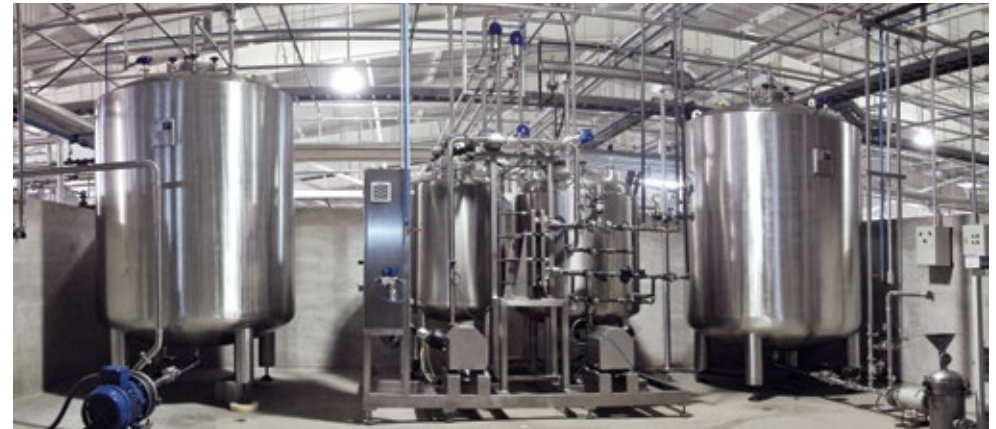
THEPROCLEAN CIP System with 2 integrated tanks and additional tanks for the PW loop. Client: Bonin / Guatemala / 2010
